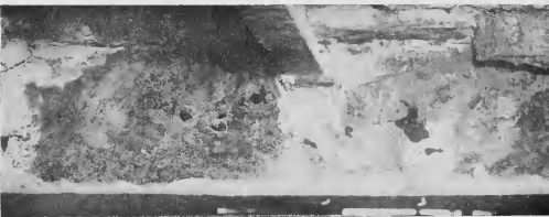
Corrosion will follow metal almost anywhere. This steel beam at the Low Octane Stillholder and Splitter plant was encased in concrete. In spite of approximately the same, however, the corrosion found its way through the concrete and attacked the steel, cutting the holes seen here. Oddly enough, other beams in the same area and under cover, were practically unharmed. An E.I.G.'s job is to find out how and why.
